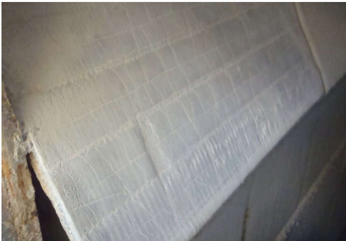
SPOT 60 OVERLAY WEAR LINERS AFER 3500 HOURS AND 8.3 MILLION TONNES
